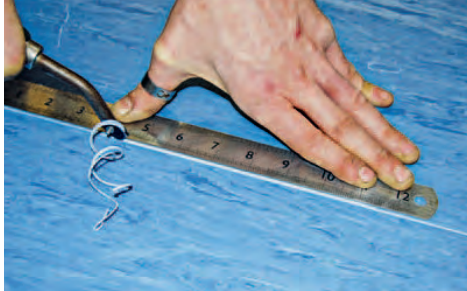
ABOVE: Care should be taken to keep the groove straight and not to groove too deep
