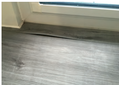
ABOVE: An issue with an LVT floor as a result of not allowing sufficient time to acclimatise the product or the adhesive not being applied right up to the edges.
