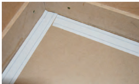
ABOVE: Direct-to-subfloor installation using mushroom tape. Use a hand roller to press the tape onto the subfloor.
