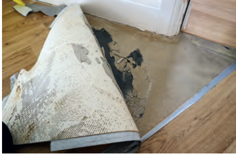
ABOVE: This sheet vinyl started to lift when the smoothing compound detached from the subfloor.
