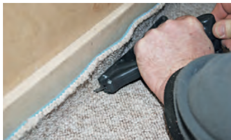
ABOVE: Using a Trim Master reduces installation time and produces a neat cut without marking the skirting.
